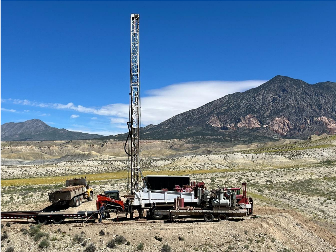
Figure 2: Picture of drill rig being set up at the Tony M Mine for the 2023 program
